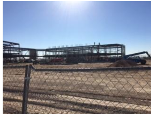
Above: Progress on the site at Lamb Blvd and Kell Ln on 11/6/16.
